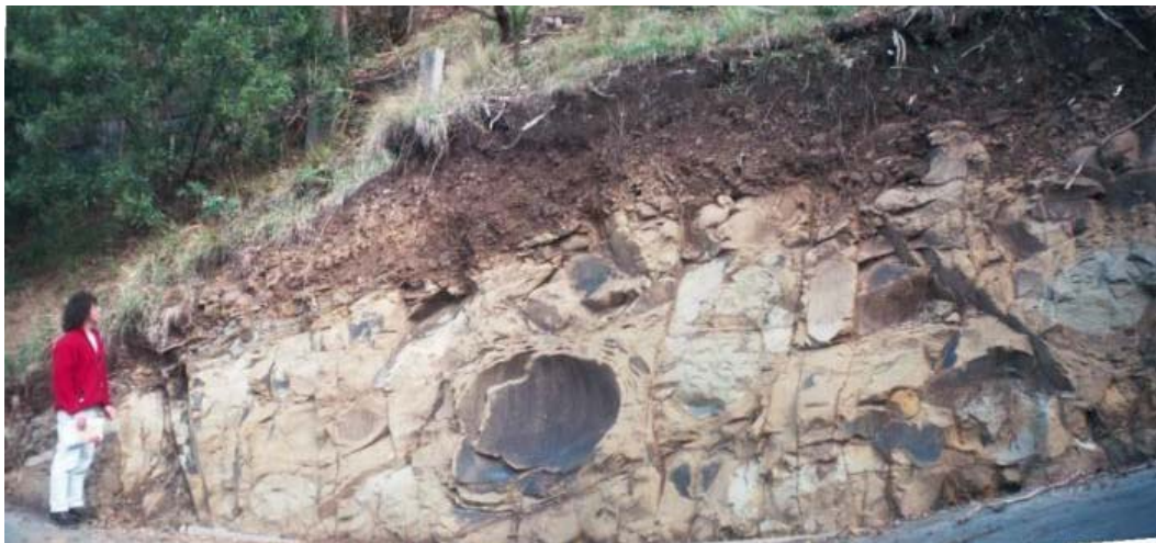
Cutting showing fractured sandstone and soil cover at Morley Avenue, Wye River
